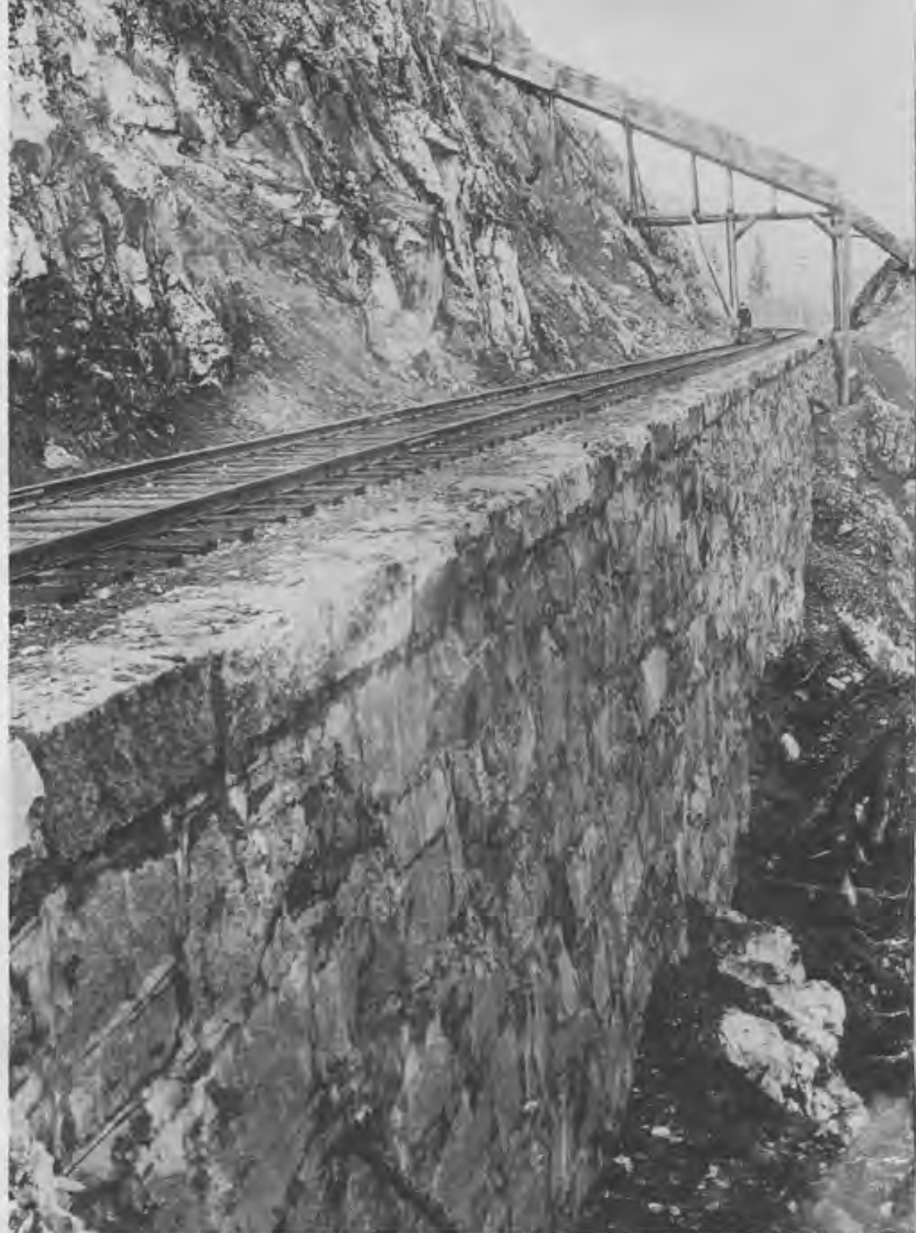
CPR masonry wall three miles west of North Bend in the Fraser Canyon.
